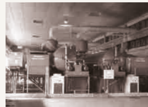
Autoclave treatment station - Moulton production site (14)
